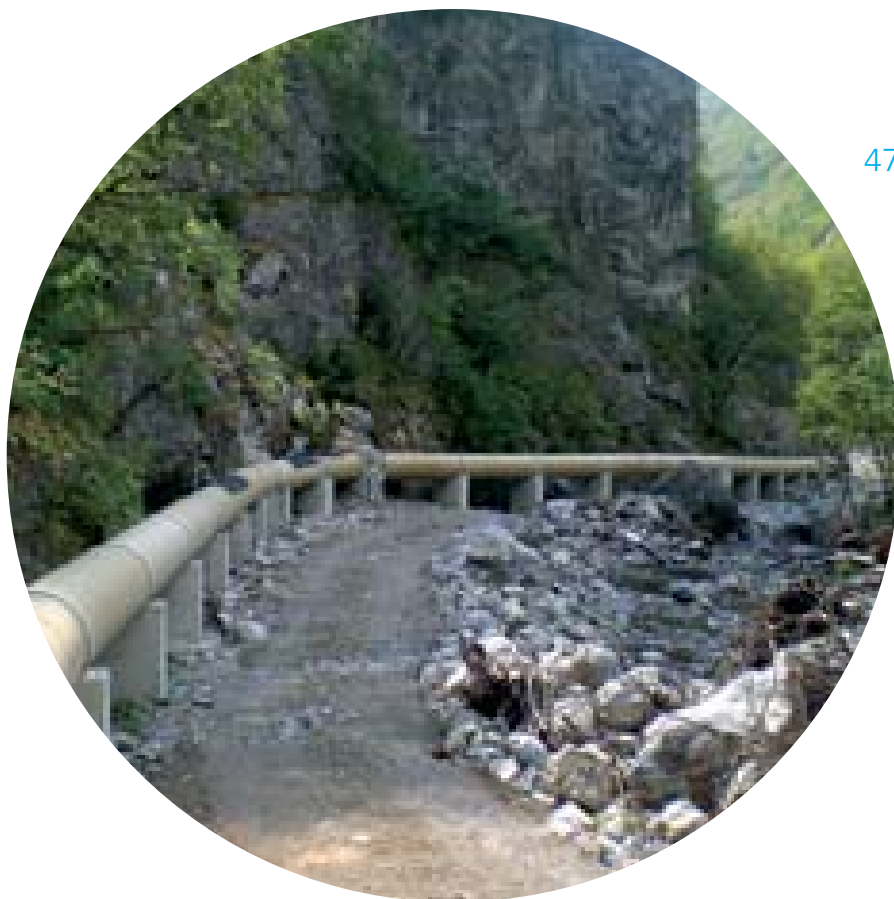
Fig. 42: Above ground installation
